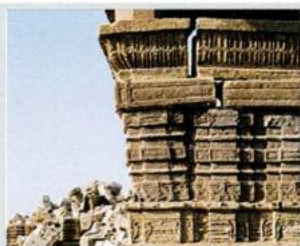
Partially Damaged Rajolati Chattri, Bhuj
