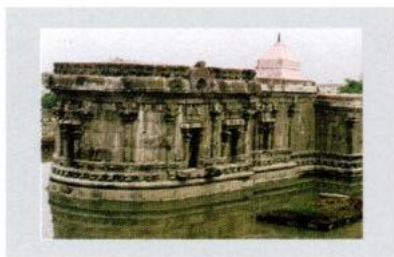
Frontal Mantapa of Amman Shrine, Pushpavaneswara Temple, Puvallakudi, Pudukkottai Dsistrict after Structural Conservation
