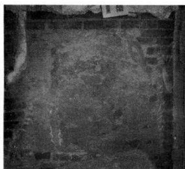
View of the Scoured out Wall After the Removal of the Sculpture
