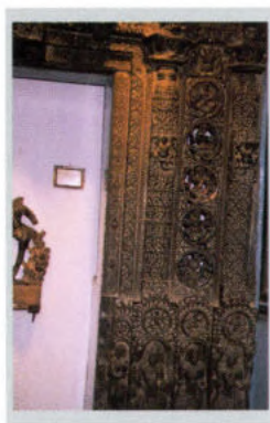
Missing Portion of the Hoysala Period Carved Stone Door and Cornices Restored Using Visually Similar Looking Wood
