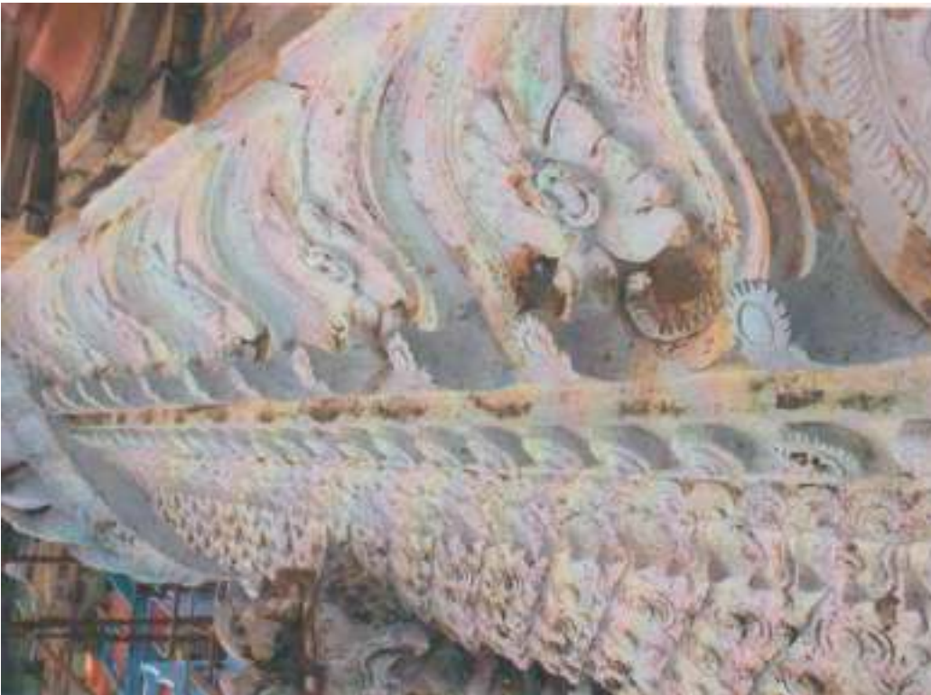
Water stagnation in the Top portion
